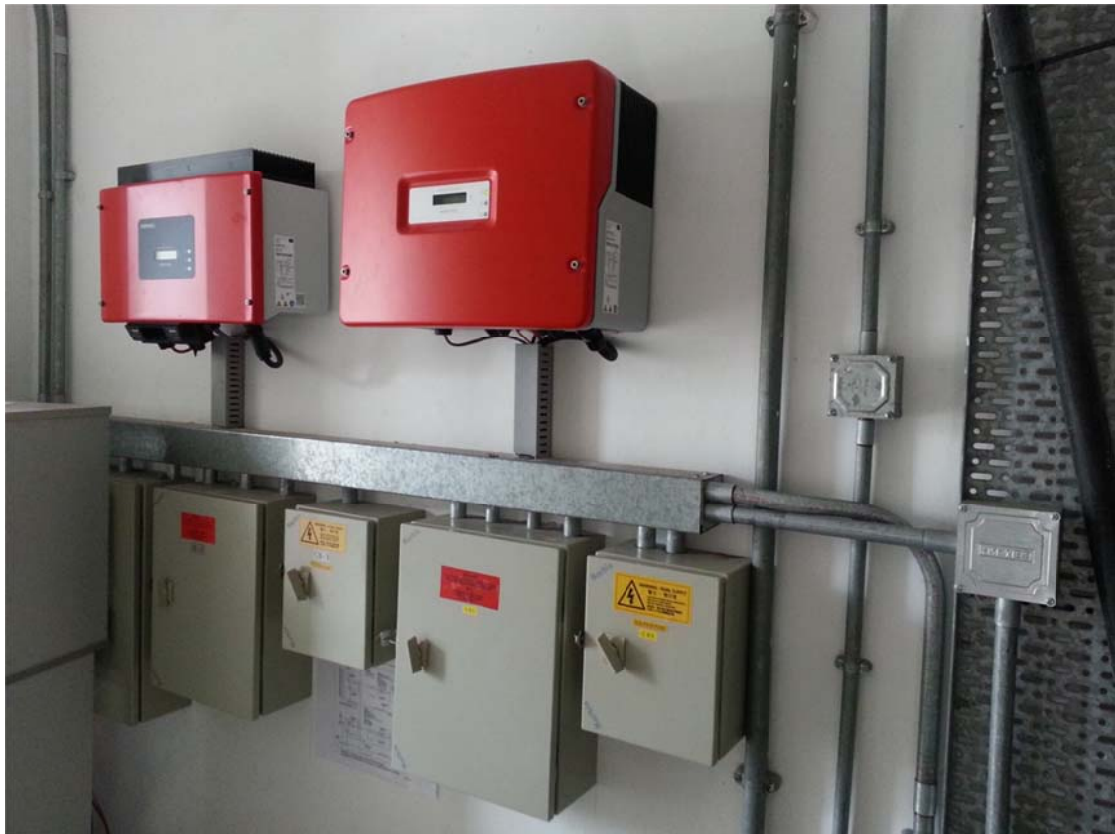
The control and protection device system was installed at the R/F plant room.
