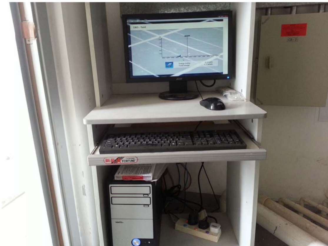
A monitoring and data logging system (BMS) was installed at the R/F plant room.
