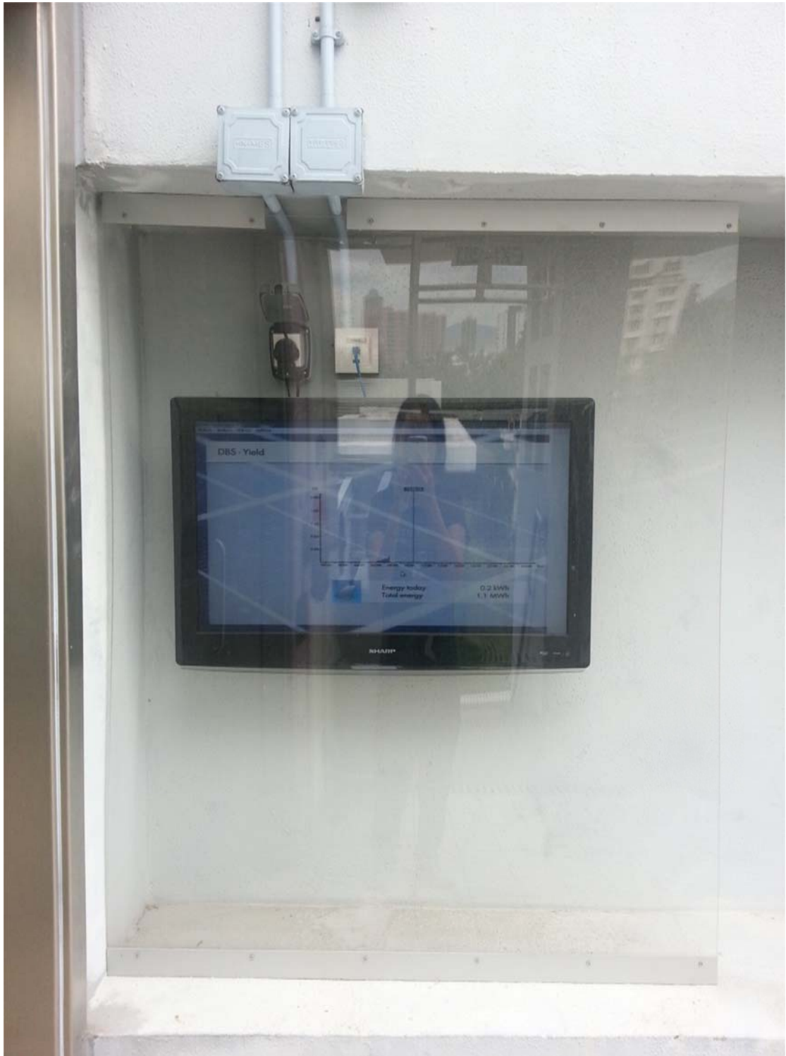
A LCD monitor was installed in the 5/F corridor.
